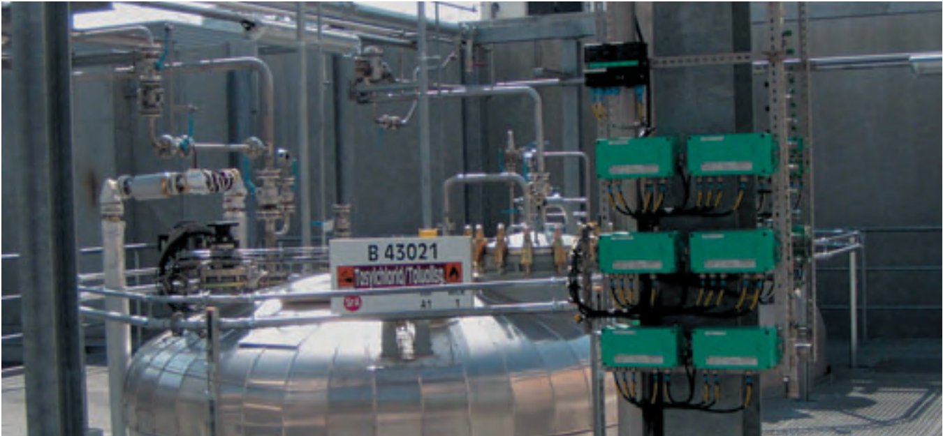
FieldConnex® from Pepperl+Fuchs in the Ketek tank farm:
